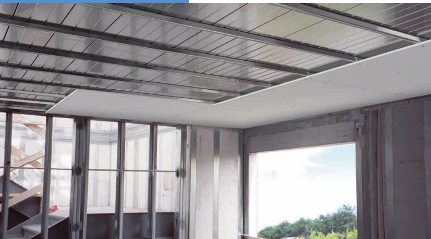
Hat Channels and Drywall
